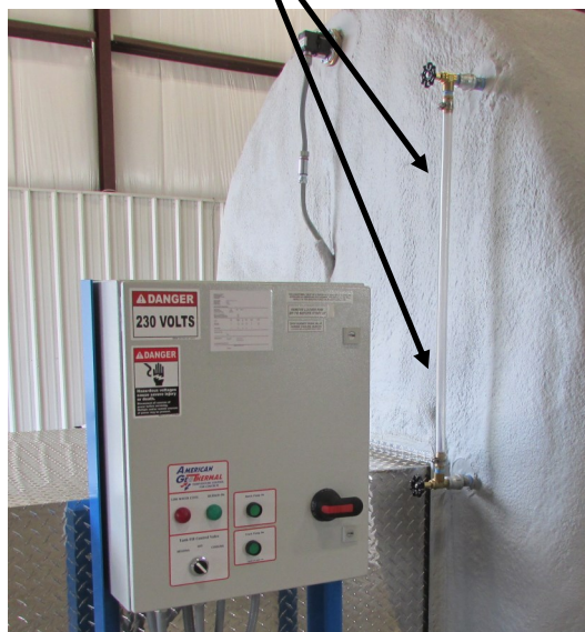
Tank Sight Tube
