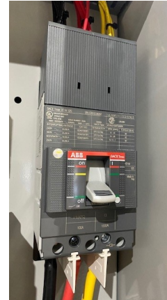
CB0, Main Chiller Breaker
