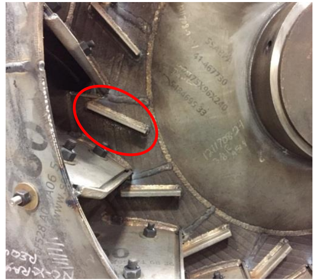
Deflector Plate on a Fan Assembly
