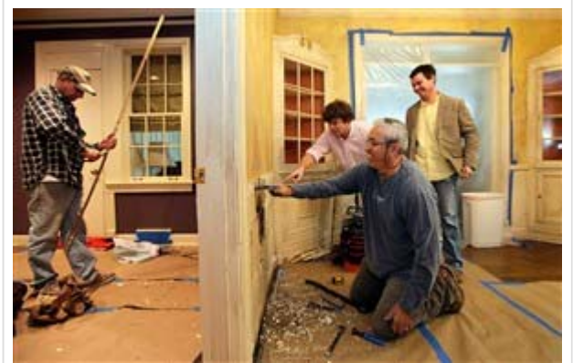
Walker Uhlhorn, top center, and George Uhlhorn, right, of Uhlhorn Brothers Construction Co., remove a plaster wall as part of a home remodeling job with carpenters John Pentz, left, and Brad Alvarez. (Photo: Lance Murphey)
