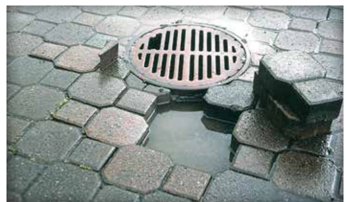
Figure 15. An absence of holes in the sides of this roof drain led to ponding.
