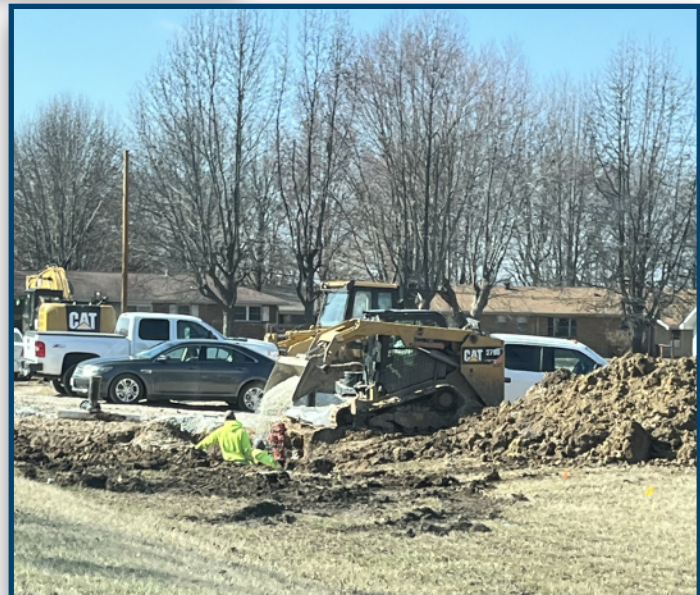
Don Maggi Construction installing new service lines to a new subdivision being built in St. James, MO.
