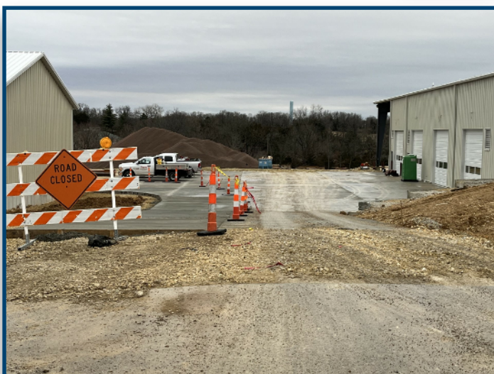
Logan Excavating finishing up concrete work on the entrance of the new Phelps County Road Department building.
