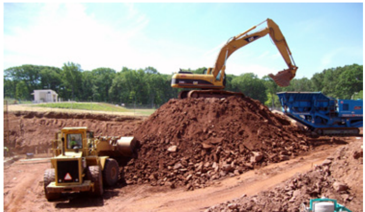
Midstate Site Development recycles rock to use as structural backfill for its other projects.
